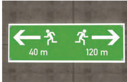
Emergency exit signs in tunnels
