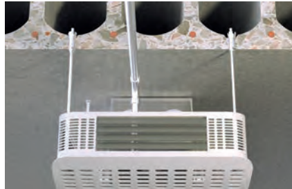
Air conditioning units in pre-stressed hollow-core concrete slabs
