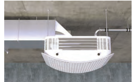
Air conditioning units
