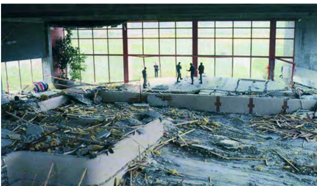
In 1985, the suspended concrete ceiling of an indoor swimming pool collapsed in Uster, Switzerland. The stainless steel ceiling attachments exhibited no external defects, but were completely destroyed internally in some cases due to stress corrosion cracking.
