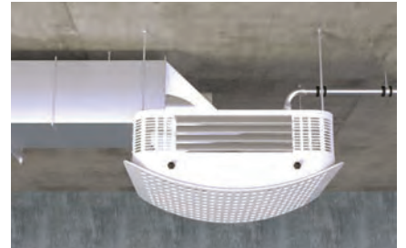
Air conditioning units
