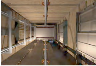
Elevator guide rails
