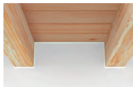
Internal expansion joints
